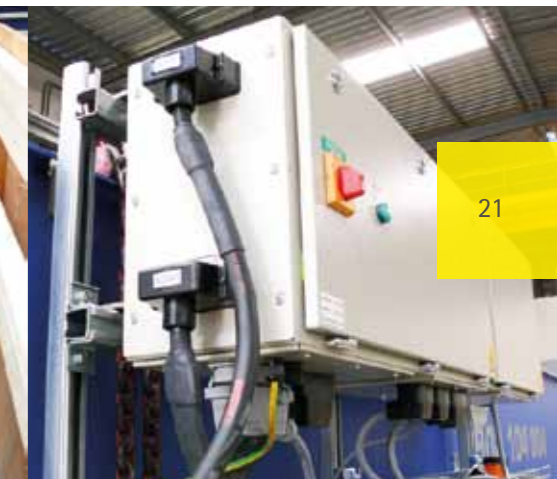
Bridge panel with plugs
