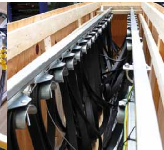
Ready to use hoist power supply
