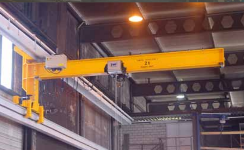
Wall console crane
